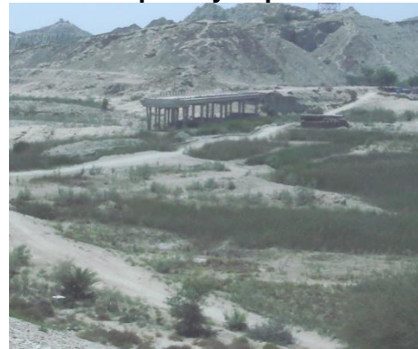
Damaged Bridge downstream of Dam
