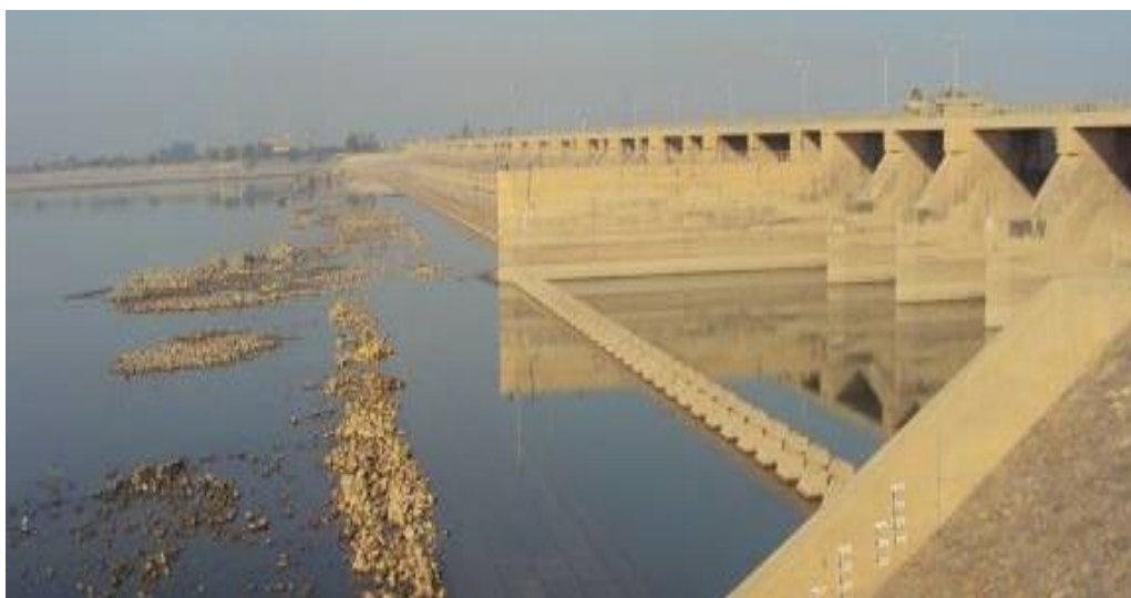
Condition of Concrete Blocks and Stone Apron after 2010 Floods
