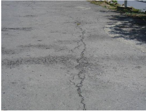
Crack on Dam Crest
